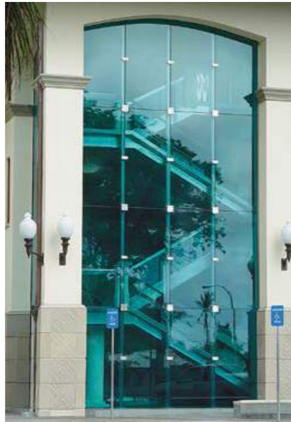
Multi tier structural stand-off system glass facade using 30.56mm thick Cyclone resistant multi-laminated glass connected to bolt through stainless steel point fixings, fixed to stainless steel full height supports behind glass.
