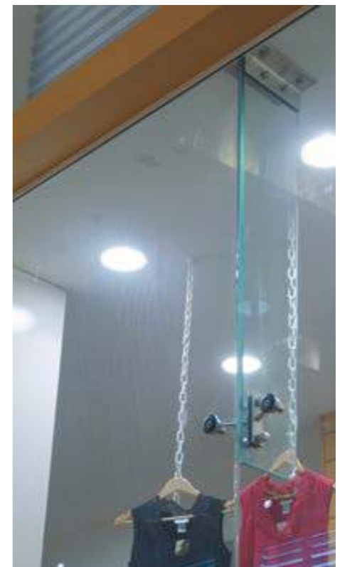
Cantilevered glass with bolt through stainless steel head mounted bracket and 2 way spider fixing for face glass connection.
