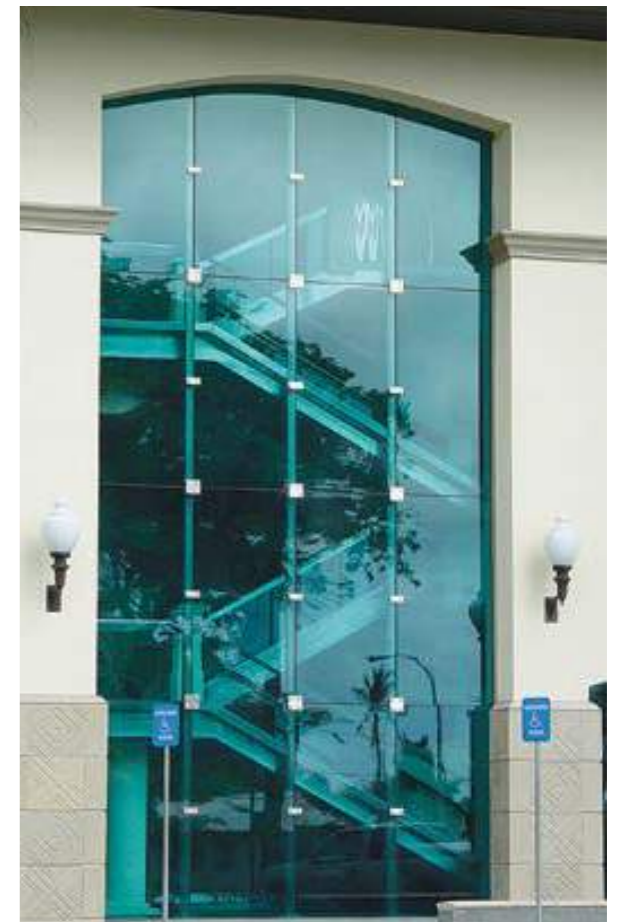
30.56mm Cyclone resistant laminated – Make-up 10mm Azuria toughened/ 2.28mm SGP/10mm clear toughened/2.28mm SGP/6mm Energy Advantage low-E (#4) toughened. Fletcher Construction American Samoa. Glazed by National Glass. Architect – Lively Architects.
