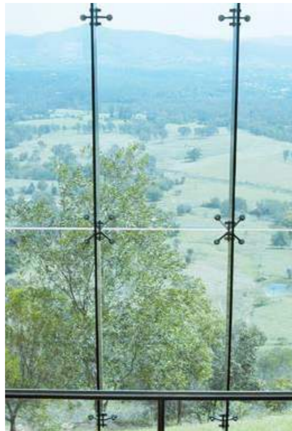
Multi tier structural stand-off system glass facade using four way spider fixing bolted off stainless steel fins – 12mm grey toughened glass .
